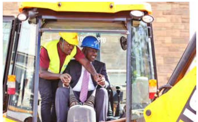
President Ruto operates a backhoe machine to break ground for the construction of i-Block
